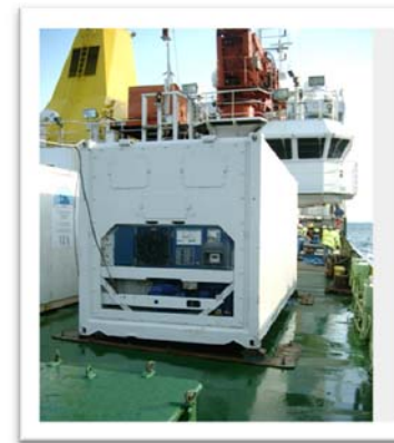
Refrigeration unit (temperature adjusted to in situ )
